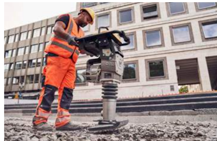
Especially on inner-city construction sites, the battery-powered rammers emit less noise and emissions and thus protect the construction site environment.
